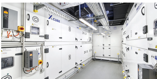
Air conditioning technology
